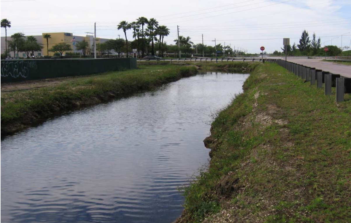
Photograph 10: (C-2 EXTENSION) East side of NW 117 th Ave just north of NW 25 th St, facing south. Shows canal banks with moderate to steep slopes, moderate to severe erosion and irregular canal width.
