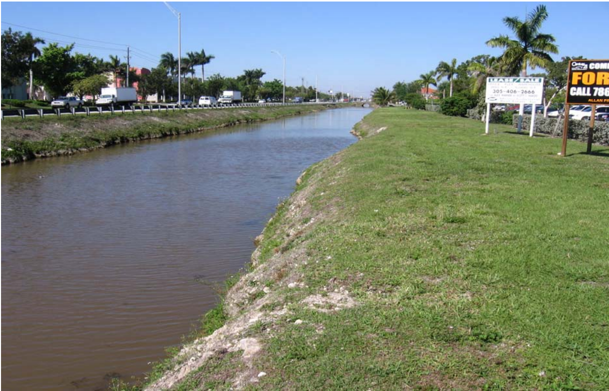
Photograph 9: (NORTHLINE CANAL) North side of NW 25 th St at intersection with NW 97 th Ave, facing west. Shows canal banks with steep slopes, moderate erosion and irregular canal width.
