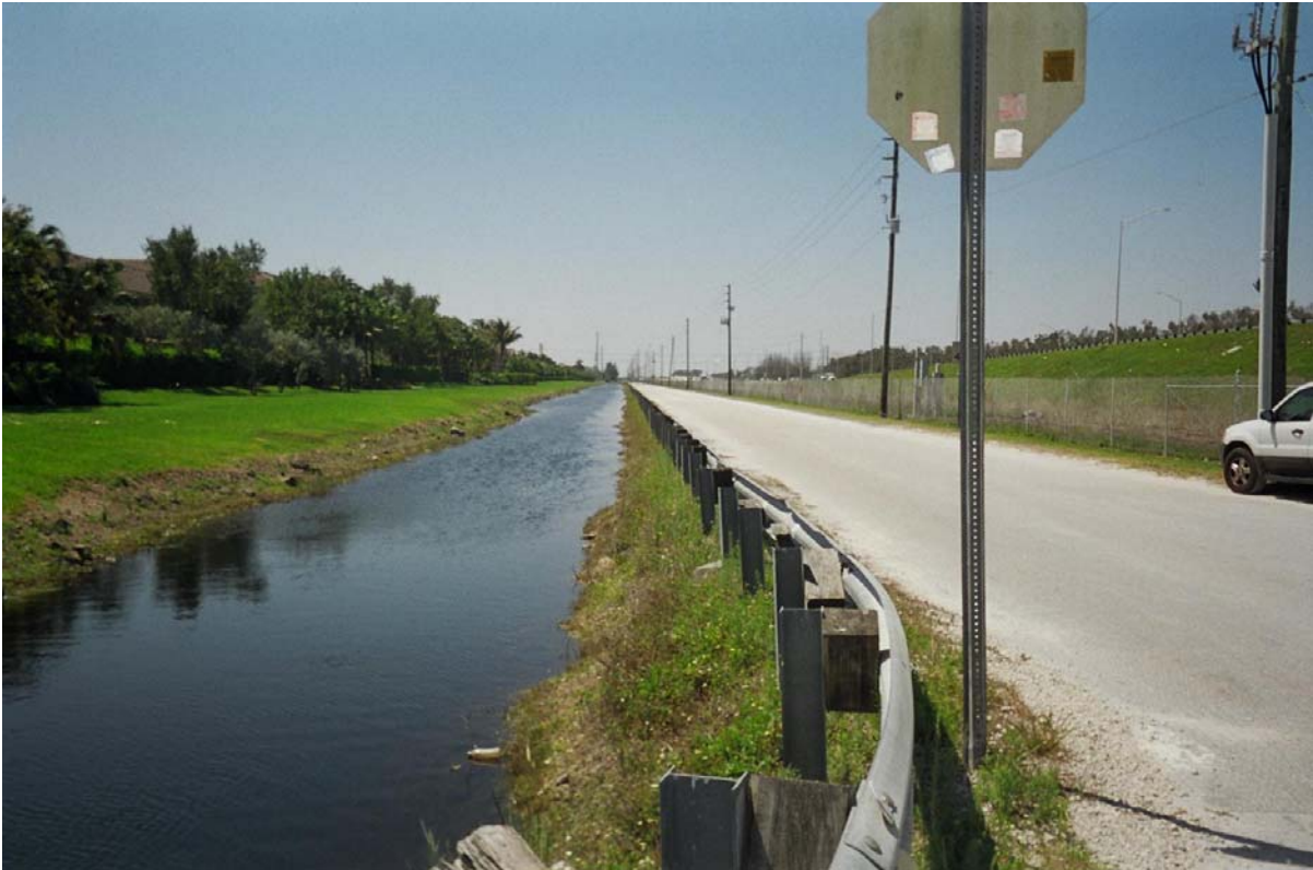
Photograph 19: (C-2 EXTENSION) Viewing south along west canal bank, shows moderate to steep canal slopes with moderate erosion, little horizontal distance between guard railing and top of bank.
