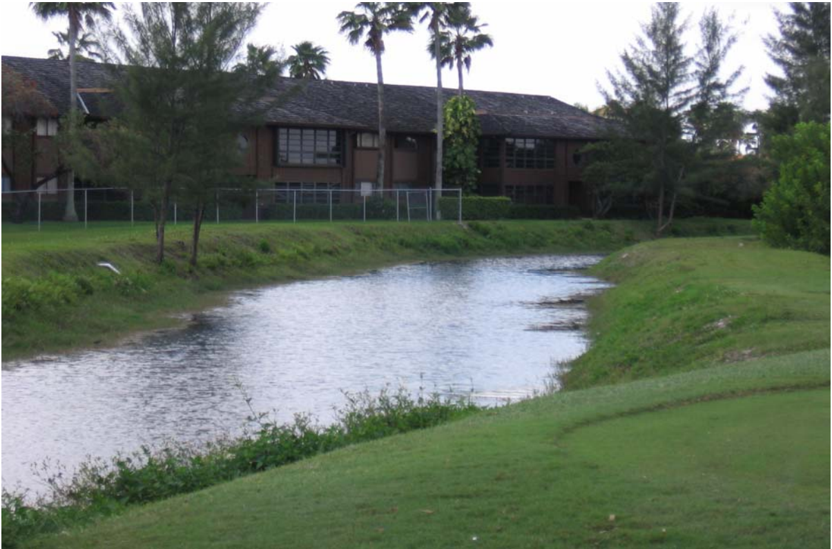
Photograph 27: (DRESSELS CANAL) Canal crossing at NW 102 nd Ave, facing west. Showing steep, grass-covered slopes with little erosion.
