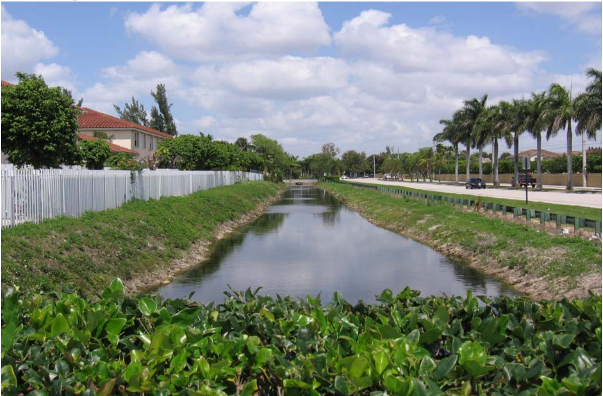
Photograph 30: (DRESSELS CANAL) West side of NW 97 th Ave just south of NW 45 th Ln, facing north. Showing moderate grass-covered slopes with little erosion.
