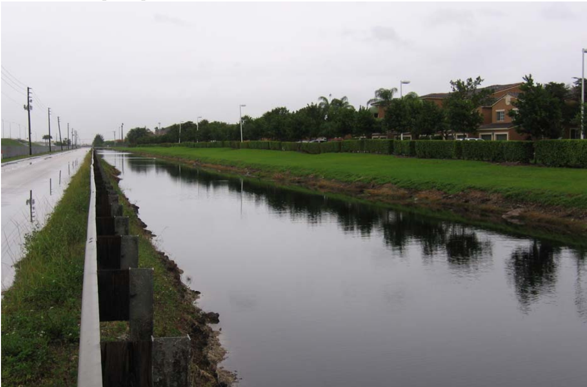
Photograph 18: (C-2 EXTENSION) East side of NW 117 th Ave just north of NW 50 th St, facing north. Shows canal banks with moderate to steep slopes and little to moderate erosion.
