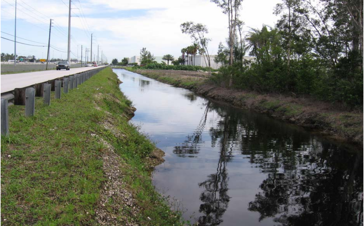
Photograph 12: (C-2 EXTENSION) East side of NW 117 th Ave just south of NW 34 th St, facing north. Shows canal banks with moderate to steep slopes, moderate to severe erosion and irregular canal width.
