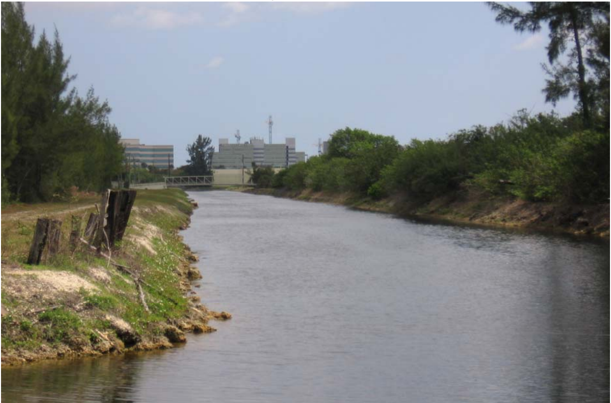
Photograph 32: (DRESSELS CANAL) Canal section along NW 40 th St, facing east. Showing moderate slopes and little to moderate erosion.
