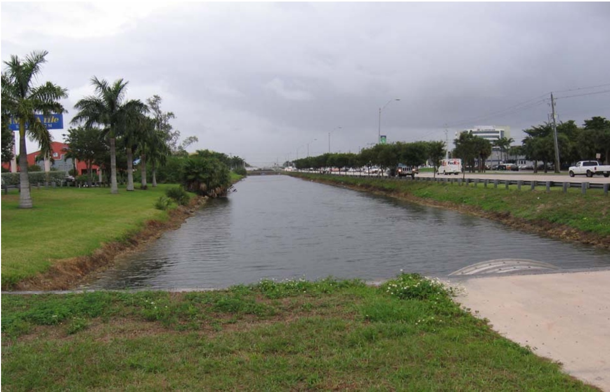
Photograph 5: (NORTHLINE CANAL) North side of NW 25 th St at intersection with NW 27 th St, facing east. Shows canal banks with gentle to moderate slopes and little erosion.
