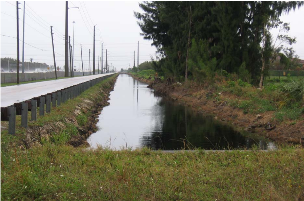
Photograph 15: (C-2 EXTENSION) East side of NW 117 th Ave just north of Doral Blvd, facing north. Shows canal banks with moderate to steep slopes and moderate erosion.
