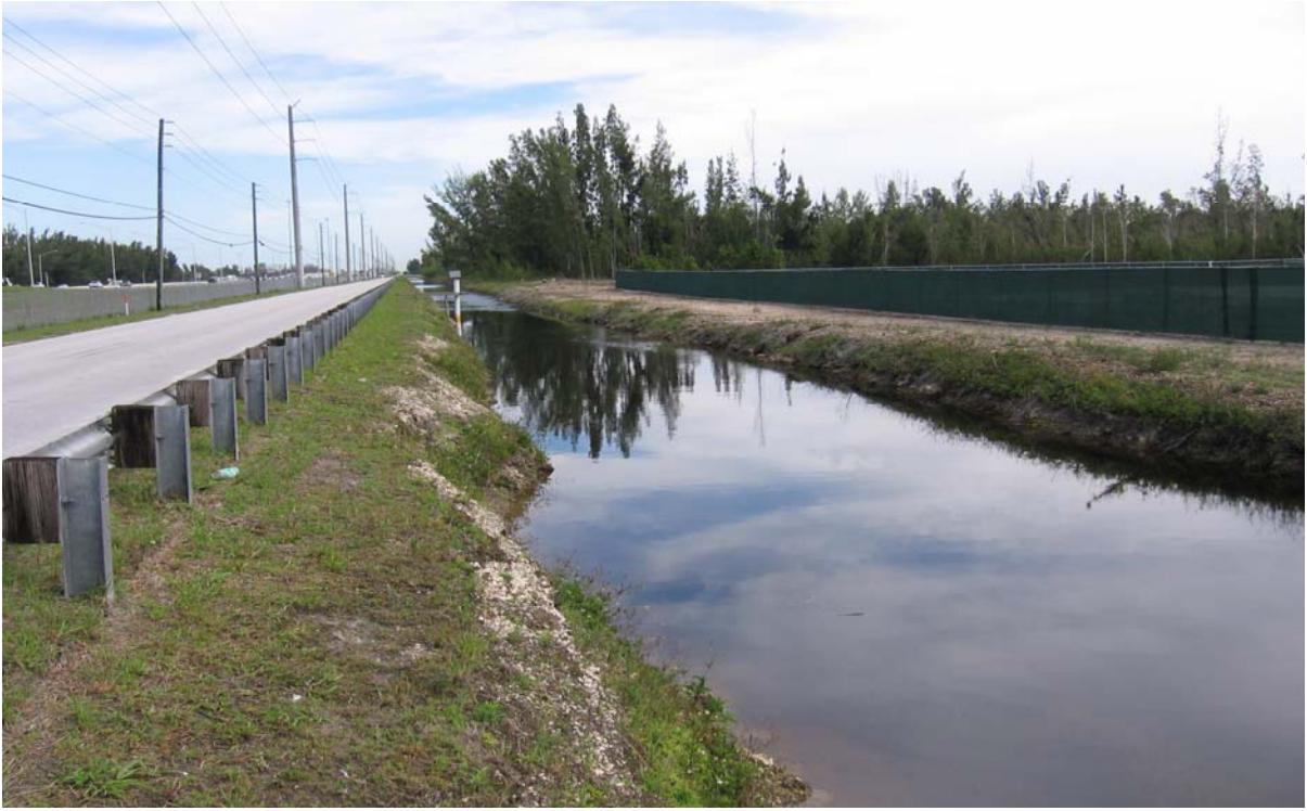
Photograph 11: (C-2 EXTENSION) East side of NW 117 th Ave just north of NW 25 th St, facing north. Shows canal banks with moderate to steep slopes, moderate to severe erosion and irregular canal width.
