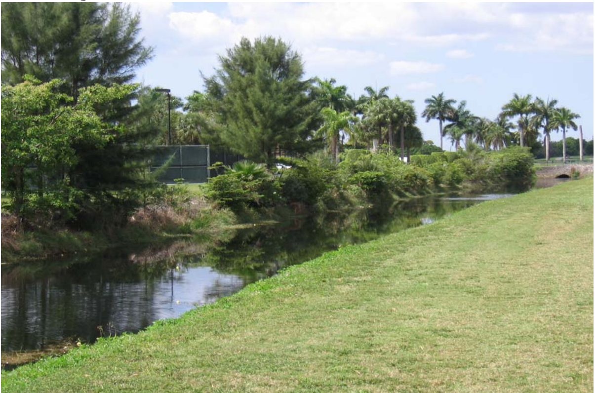
Photograph 26: (DRESSELS CANAL) Canal section between NW 104 th Ave and NW 102 nd Ave, facing southwest. Showing heavy overgrowth along south bank.
