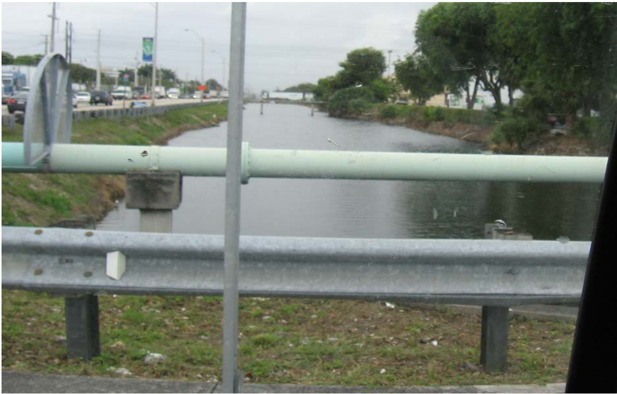
Photograph 3: (NORTHLINE CANAL) North side of NW 25 th St at intersection with NW 79 th Ave, facing west. Shows canal banks with moderate slopes and little erosion.
