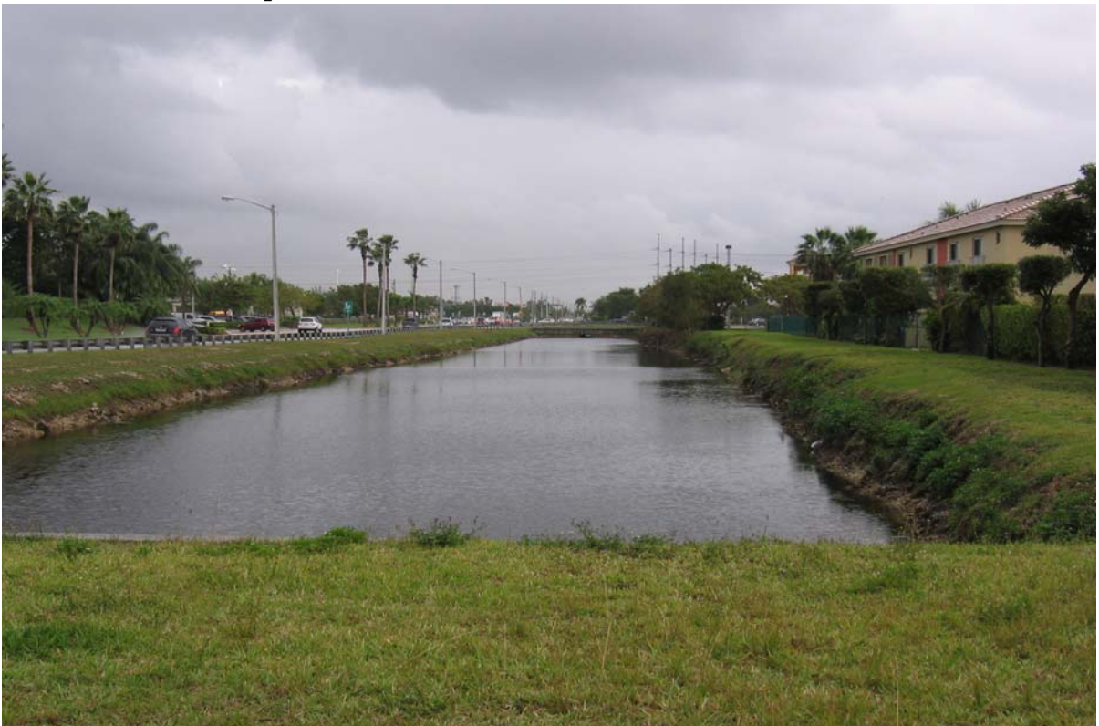
Photograph 22: (DRESSELS CANAL) NW 109 th Ave at intersection with NW 58 th St, facing east. Shows canal banks with moderate to steep slopes and moderate erosion.
