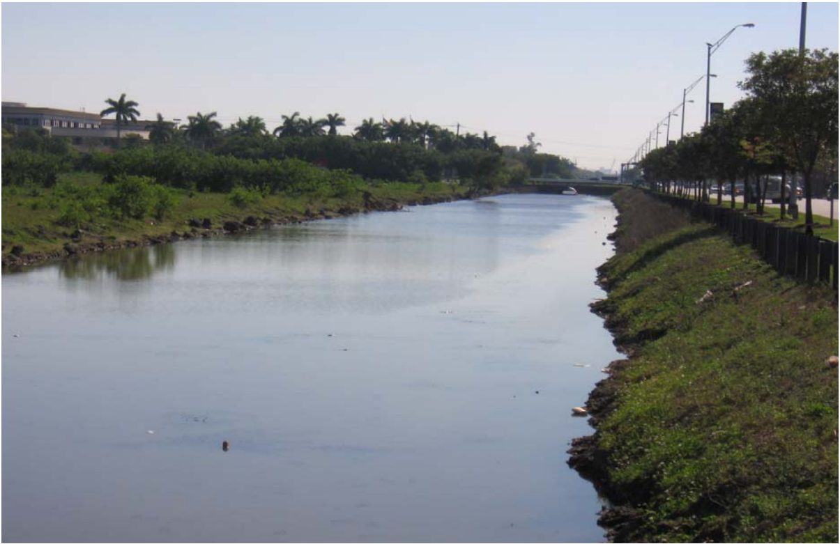
Photograph 7: (NORTHLINE CANAL) North side of NW 25 th St at intersection with NW 94 th Ave, facing east. Shows canal banks with gentle to moderate slopes and little erosion. Numerous boulders visible along northern canal bank.
