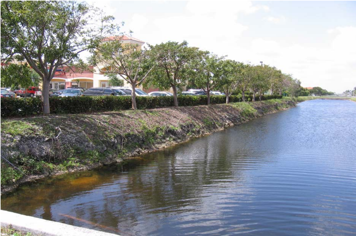
Photograph 23: (DRESSELS CANAL) NW 58 th St just west of NW 107 th Ave, facing west. Showing steep slopes and severe erosion on south canal bank (adjacent to "Delia Plaza").
