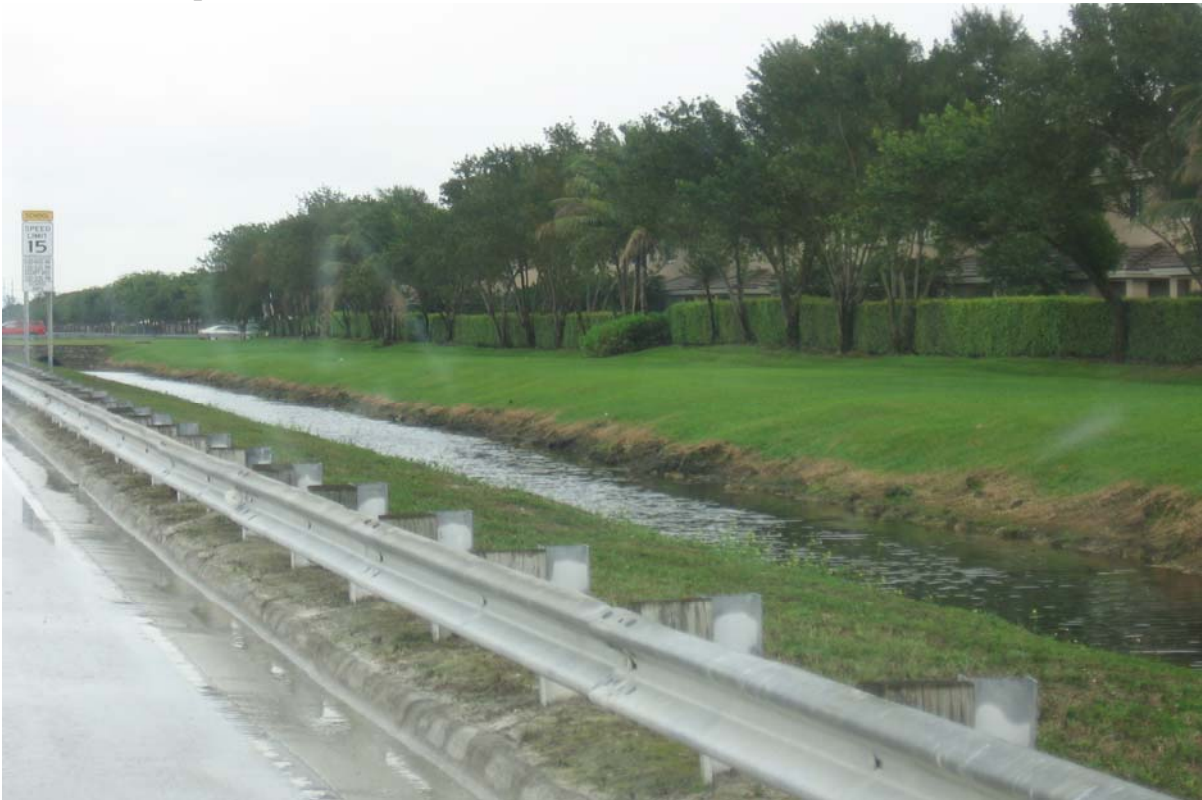
Photograph 20: (DRESSELS CANAL) South side of NW 58 th St just east of NW 112 th Ave, facing southwest. Shows canal banks with moderate slopes and little to moderate erosion.
