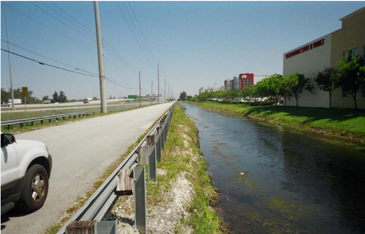
Photograph 13: (C-2 EXTENSION) Viewing north along west canal bank, shows moderate to steep canal slopes with moderate erosion, little horizontal distance between guard railing and top of bank.
