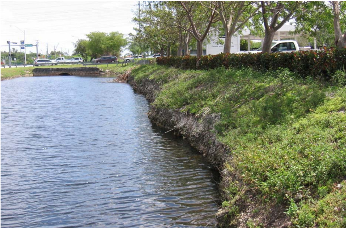
Photograph 24: (DRESSELS CANAL) NW 58 th St just west of NW 107 th Ave, facing east. Showing steep slopes and severe erosion on south canal bank (adjacent to "Delia Plaza").
