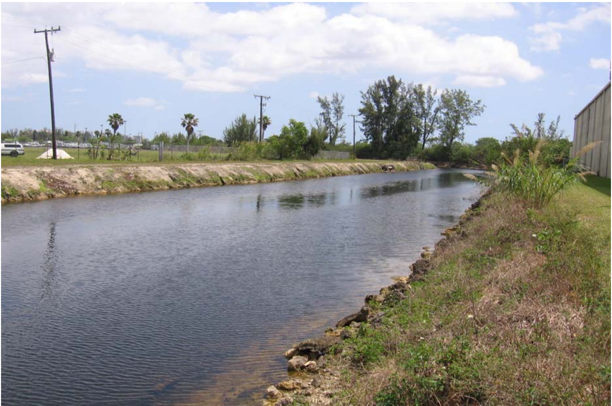
Photograph 31: (DRESSELS CANAL) Canal section along NW 40 th St, showing moderate slopes and little to moderate erosion. Also numerous boulders along west bank.
