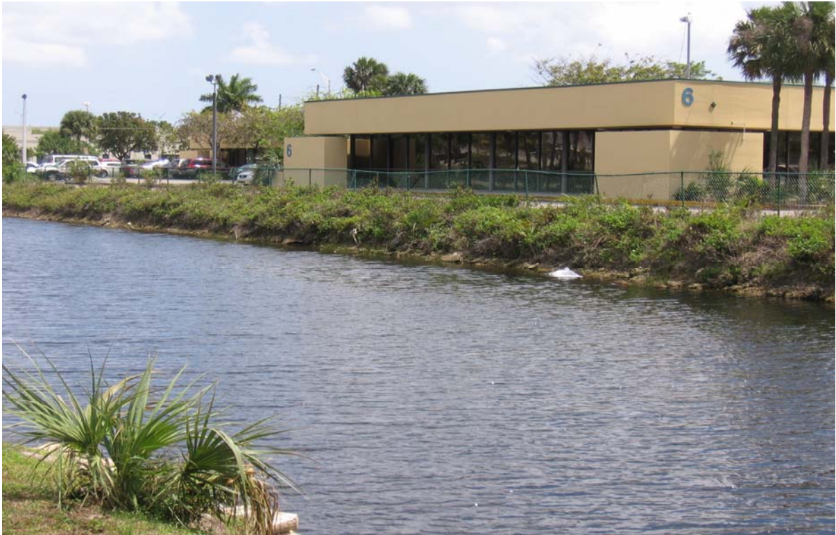
Photograph 35: (DRESSELS CANAL) NW 41 st St just west of NW 79 th Ave, facing southeast. Showing moderate to severe erosion and heavy overgrowth.
