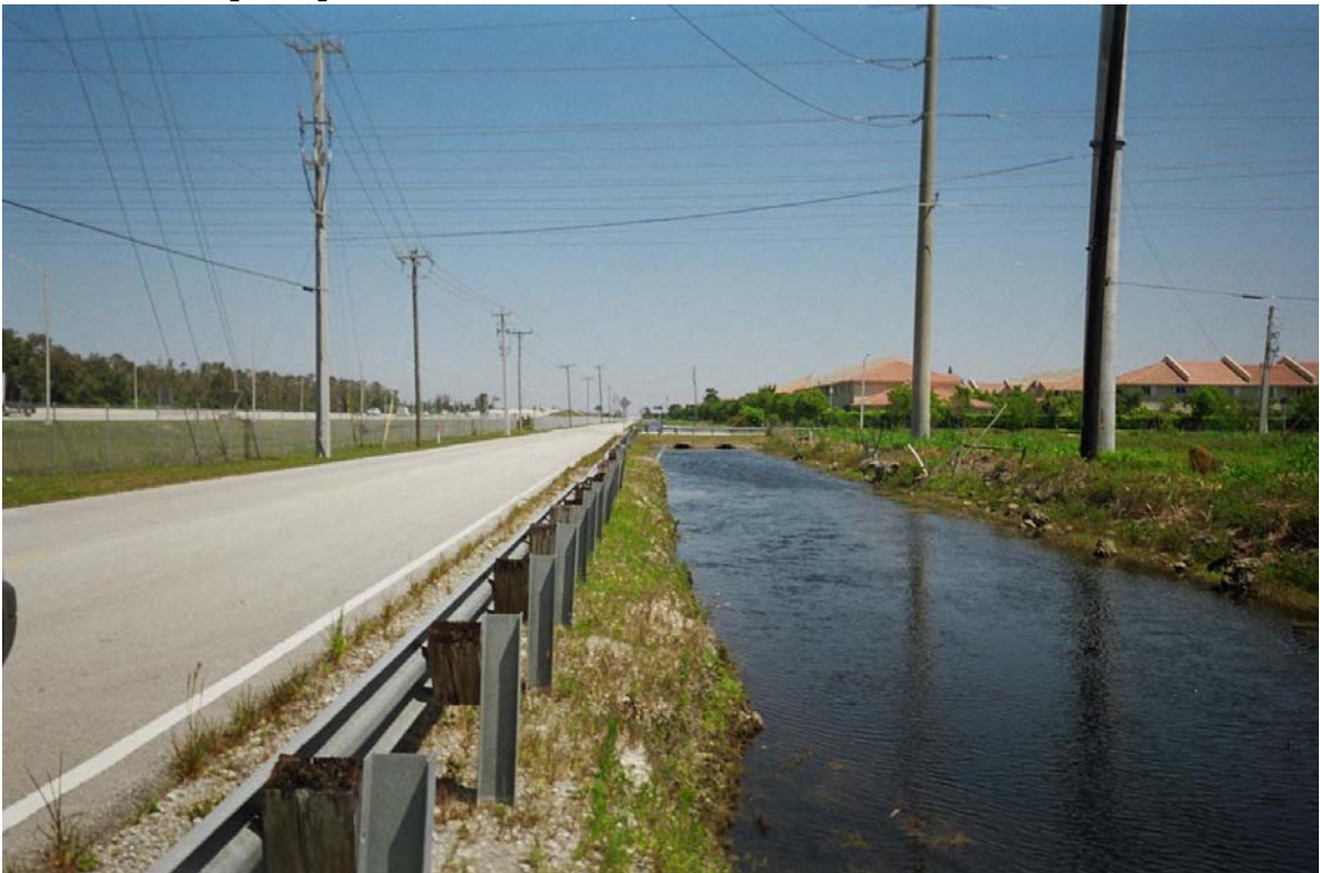
Photograph 16: (C-2 EXTENSION) Viewing north along west canal bank, shows moderate to steep canal slopes with moderate erosion, little horizontal distance between guard railing and top of bank.
