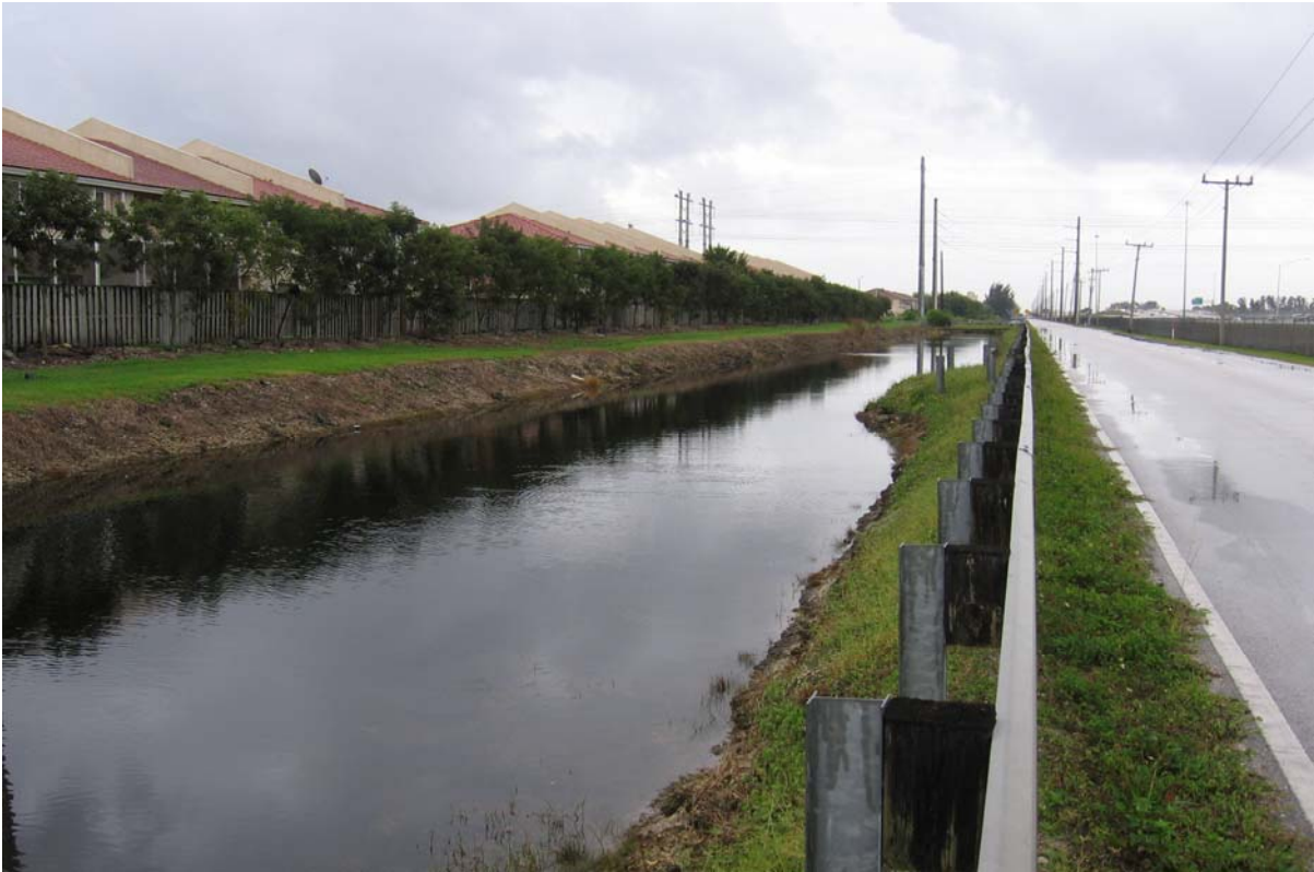
Photograph 17: (C-2 EXTENSION) East side of NW 117 th Ave just north of NW 50 th St, facing south. Shows canal banks with moderate to steep slopes and moderate erosion.
