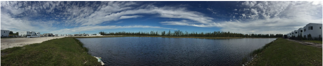
Figure 2.58: Panoramic view of the lake at Doral Glades Park during construction in February 2016.
